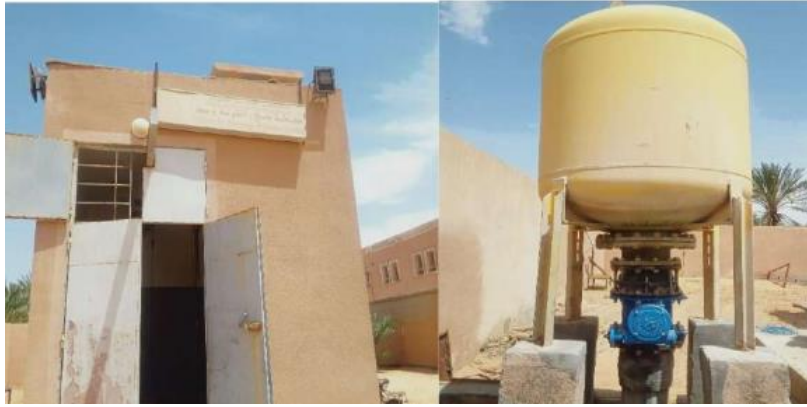
Figure III.13 Station de pompage
