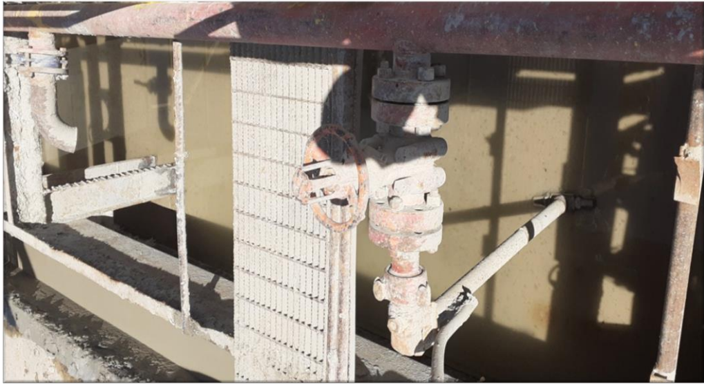
Figure II.14: bac à boue. [02]
