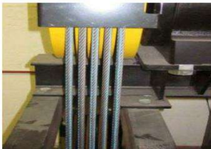
Figure I-16 : Câbles de traction.
