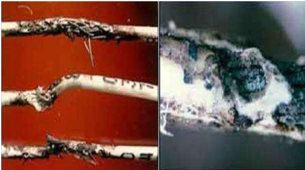
Figure I.20. Cable overheating faults.
