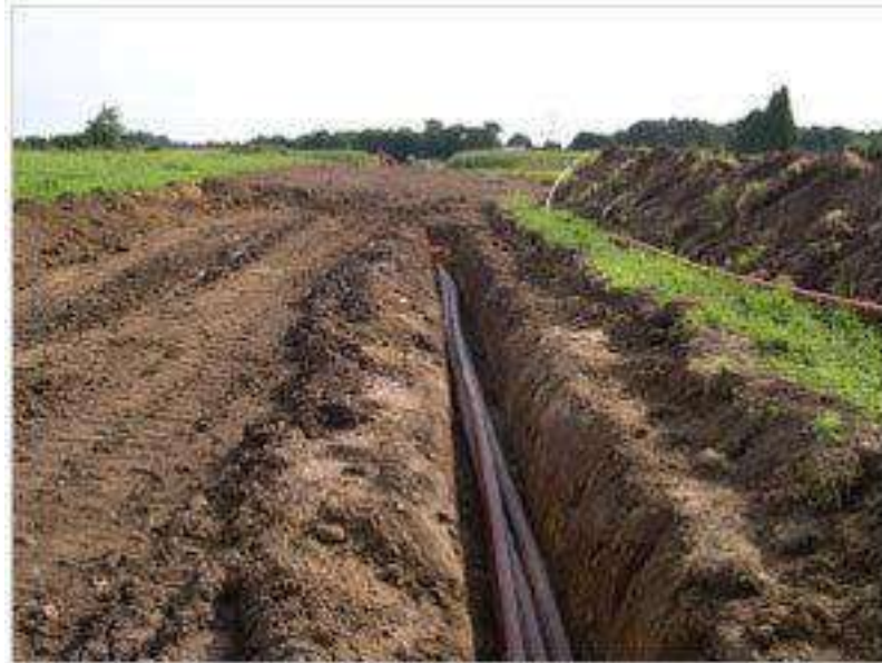
Figure I.4. Underground transmission lines.
