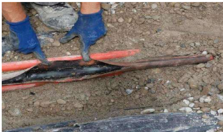
Figure I.19. Locally damaged cables (EDF image) [20].
