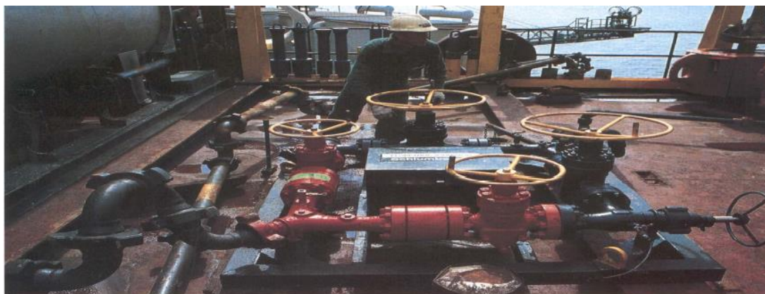
F.3.2- (Choke manifold)
