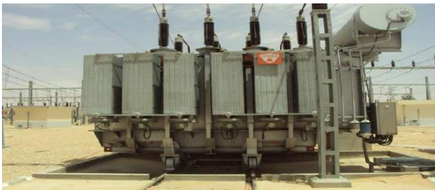
Figure 2.1 Power Transformer (GRET OUARGLA)
