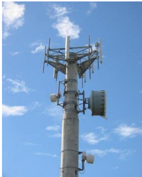
Figure I.4 :Exemple d'antenne GSM (BTS tri-sectorielles)
