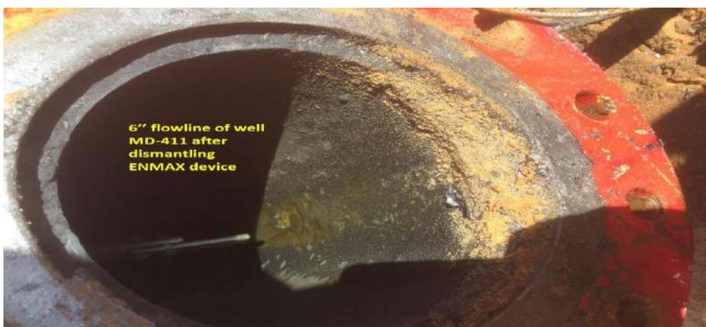
Figure III.98: 6'' flowline of well MD-411 downstream of NMAX device after dismantling the device.
