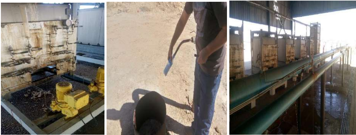
Figure I.33: dosing pump Figure I.34: sampling valve Figure I.35: inhibitor injection line
