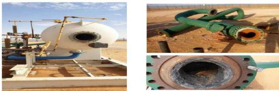
Figure I.20 : BaSO 4 deposits in the separation centre.
