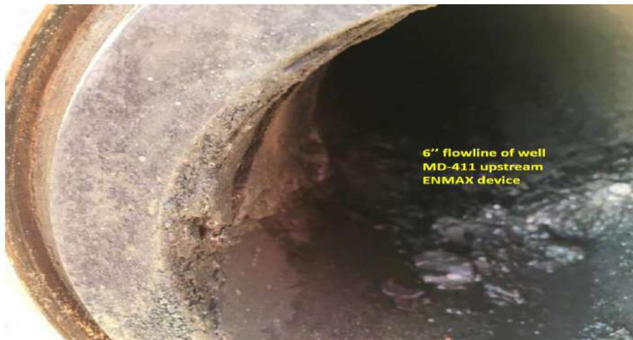
Figure III.99: 6'' flowline of well MD-411 upstream of NMAX device after dismantling the device.
