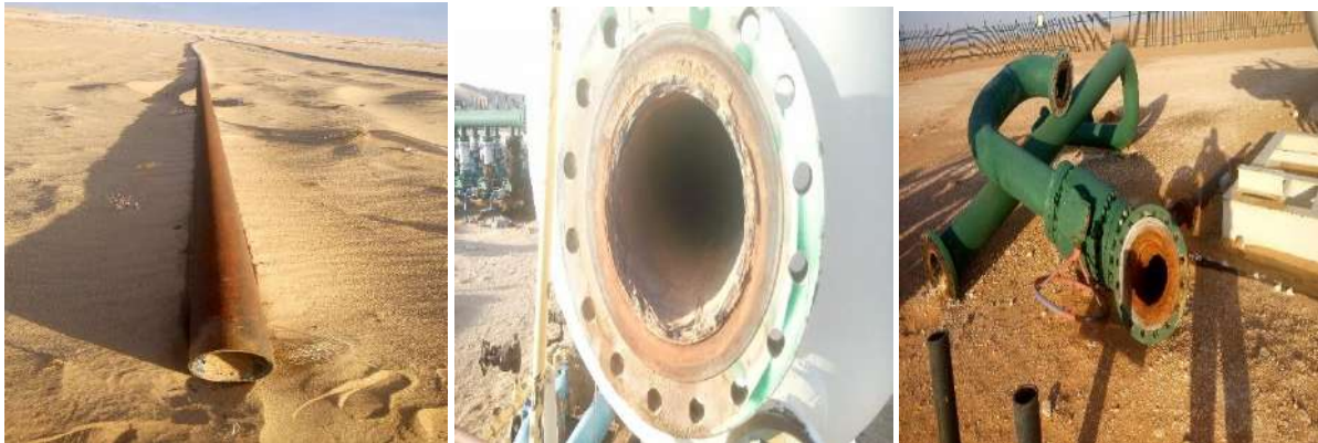
Figure I.16: Deposits of BaSO 4 in the field of Hassi Messaoud.
