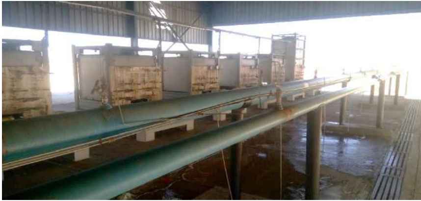
Figure I.29: system of injecting inhibitors in CIS station (HMD field).
