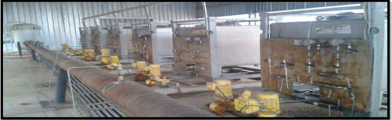
Figure I.32: Z14 station tanks
