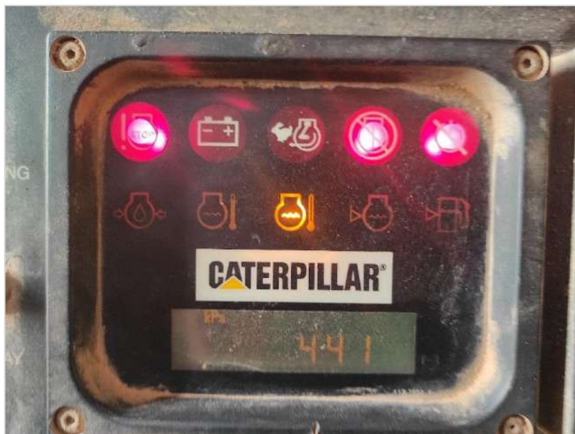
Figure 3-2 : Cat 3512B control panel showing multiple warnings
