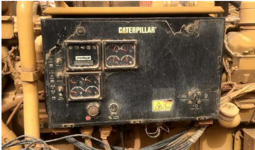
Figure 3- 9 : A malfunctioned 3512B generator at the DMP for diagnosis
