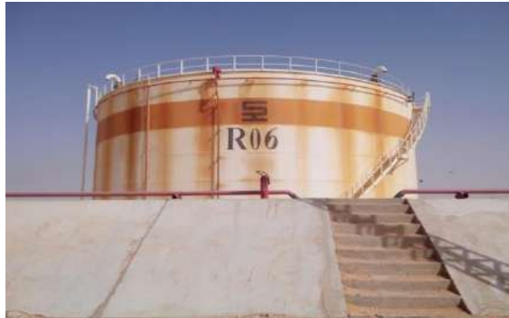
Figure 17 Oil storage tank R-06
