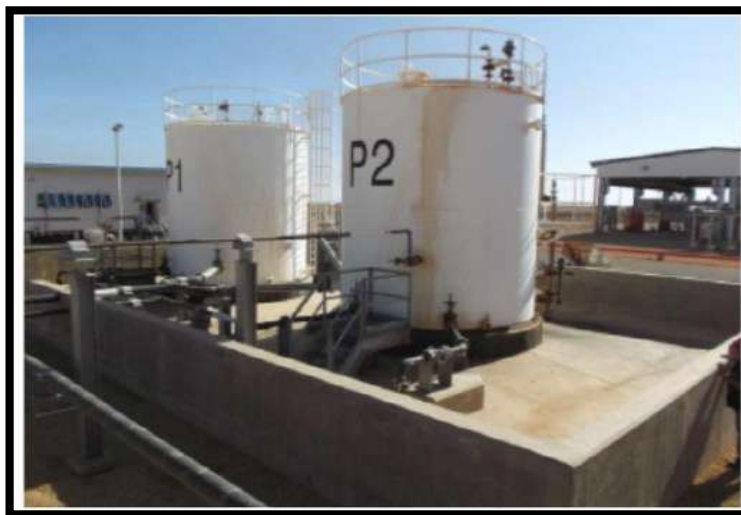
Figure III.19: Slop Oil storage tank P1/P2- WTC/NMWIC
