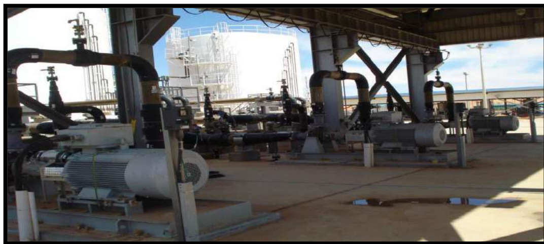
Figure III.14: Water Lift Pumps (CTE-PA-44-01A/B/C).
