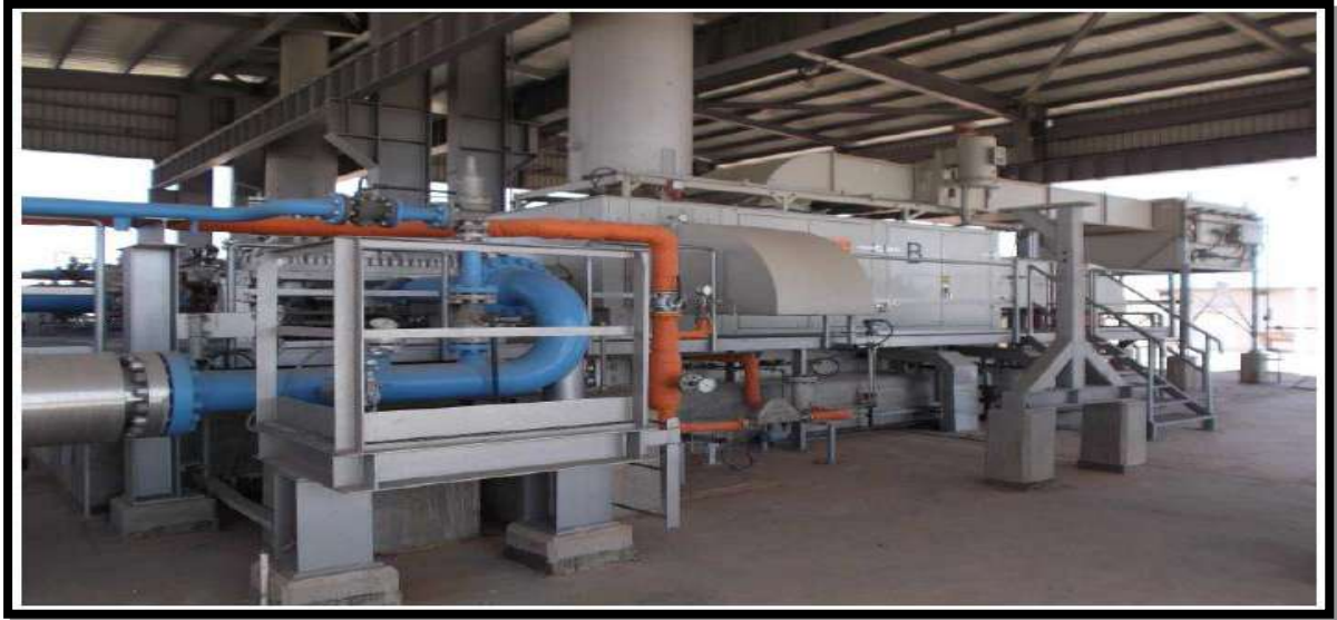
Figure III.21: Injection water turbopump WTC/NMWIC.
