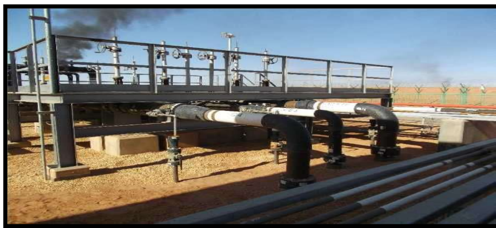
Figure III.13: Inlet Manifold WTC/NMWIC.
