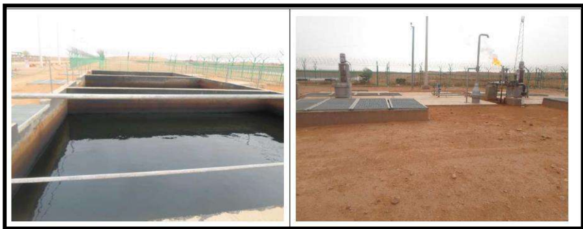
Figure III.20: Sludge drying beds WTC/NMWIC
