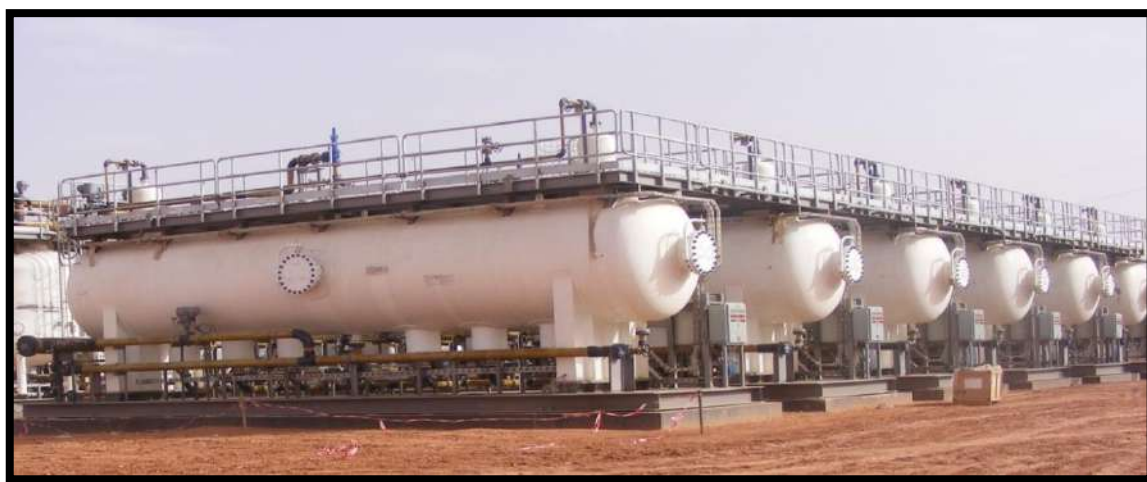
Figure III.15: Gravity separators (CTE-VA-44-01A/B/C/D/E/F).
