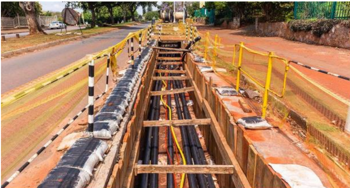
Fig I. 17 Underground HTA cable
