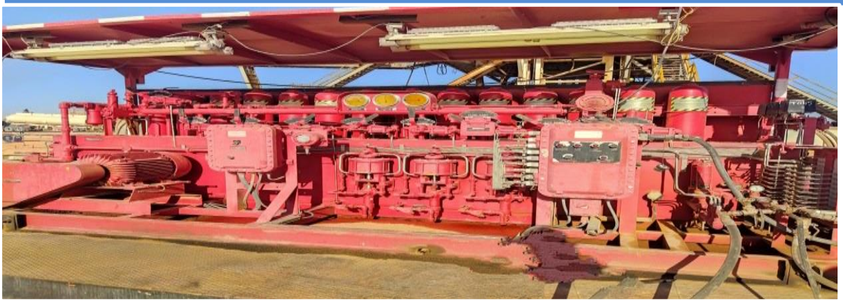
Figure II.21. real picture of BOP control system (Koomey)
