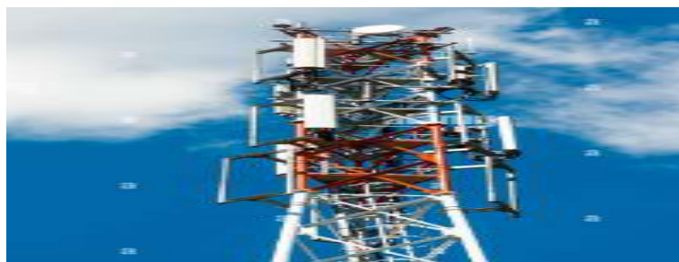
Figure 4 : Station de base (SB).
