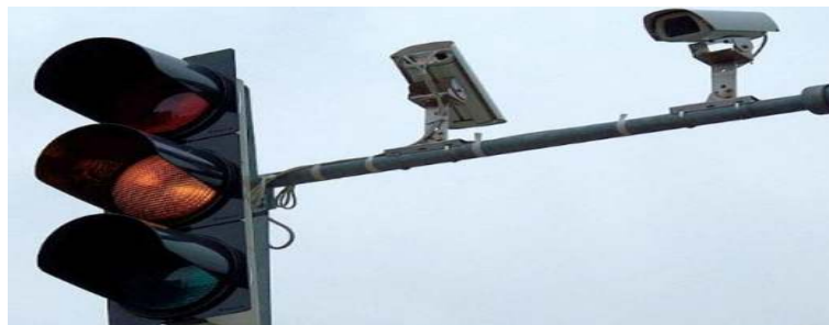
Figure 3: Road Side Unit.
