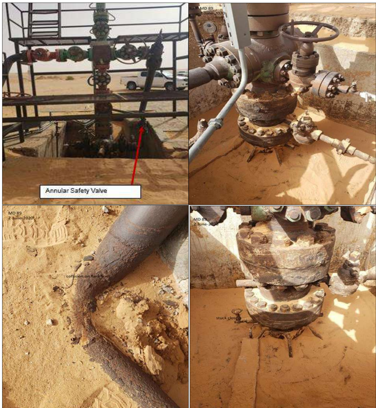
Figure III.12: MD-89 Wellhead Situation
