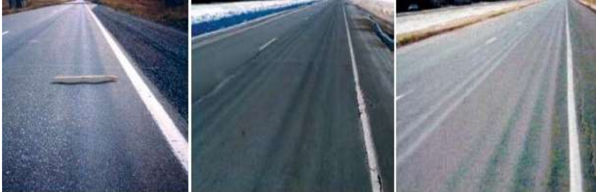
Figure 2: Examples of Rutting at different Severity Levels
