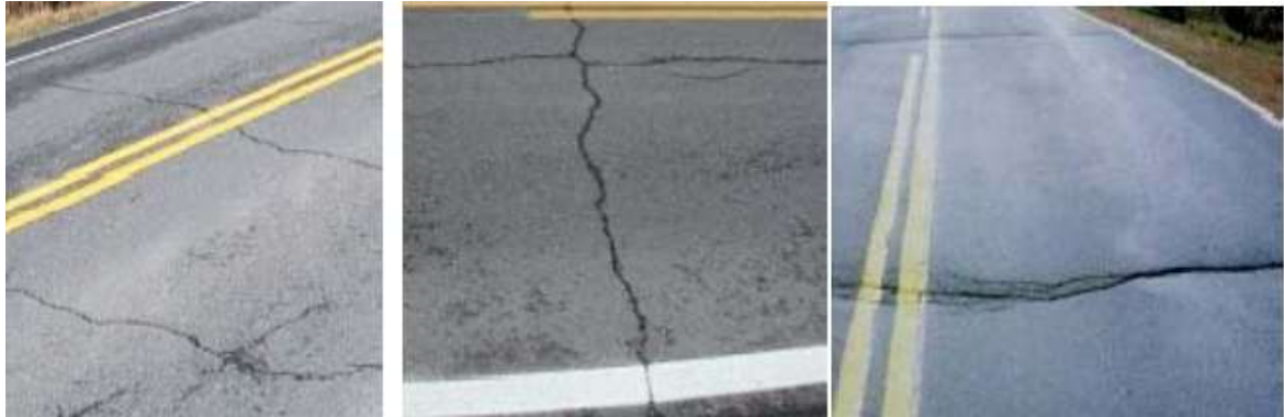
Figure 3: Examples of Cracking at Different Severity Levels.
