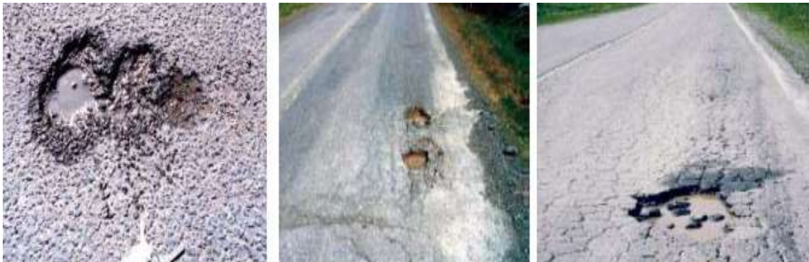
Figure 1 : Examples of Potholes at different Severity Levels.
