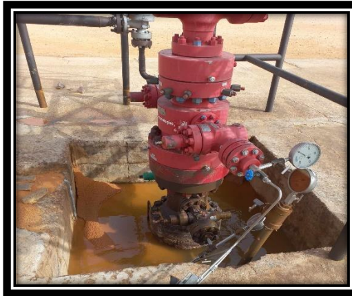
Figure I.11: Electrochemical corrosion in wellhead.
