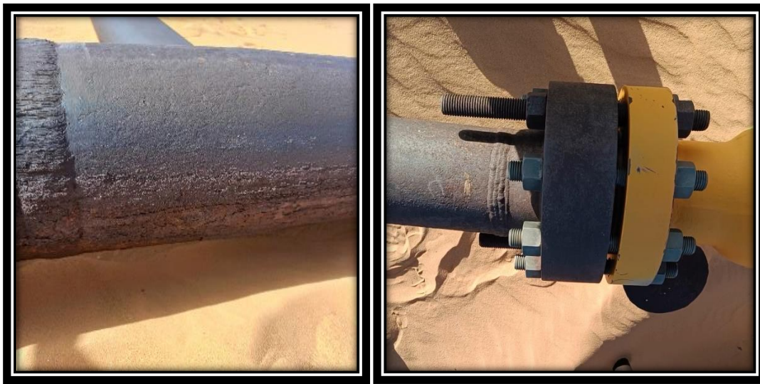
Figure III.1: corroded parts of the injection system
