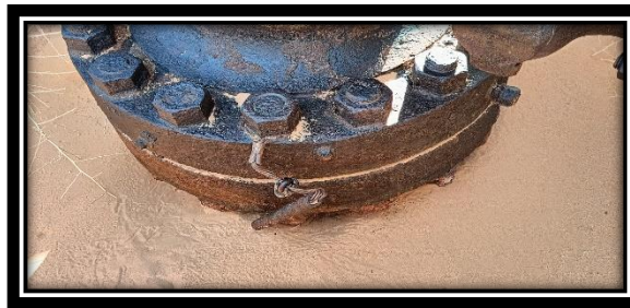
Figure I.10: Chemical corrosion in wellhead.
