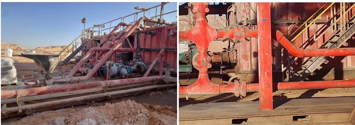
Figure II.1: 45° elbows in drilling rig
