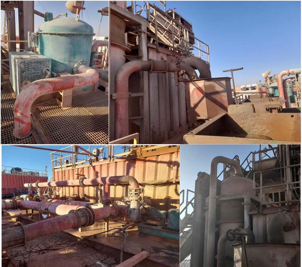
Figure II.2: 90° elbows in drilling rig
