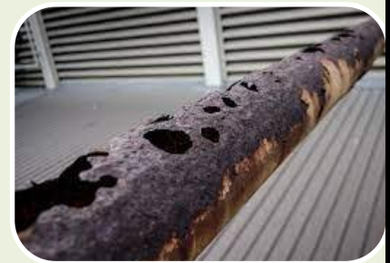
Inter Granular Corrosion
