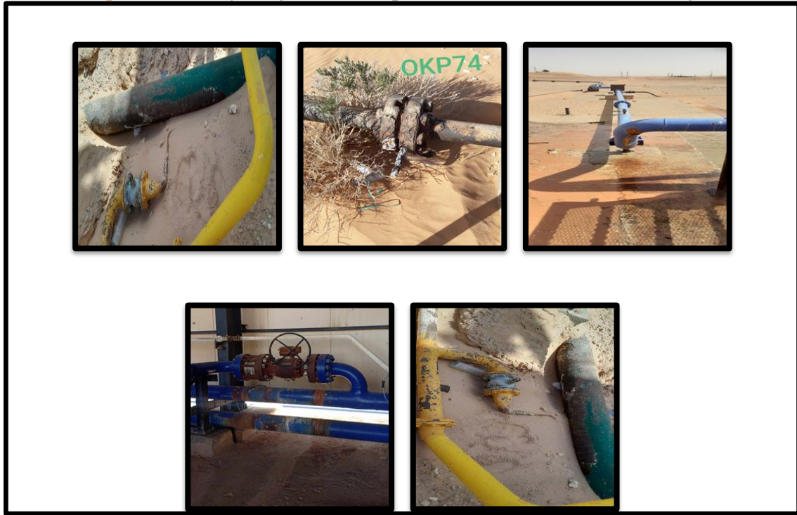
Figure II-3 : Corrosion of Above-Ground Production Installations
