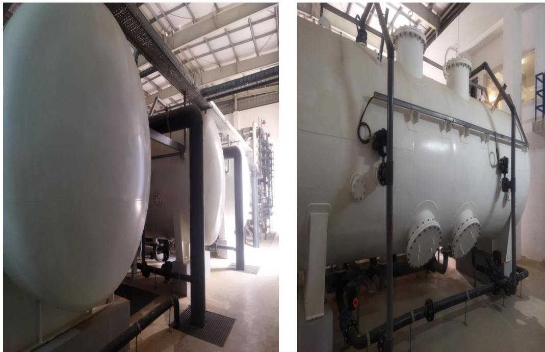
Figure II-6 : Sand Filter Units
