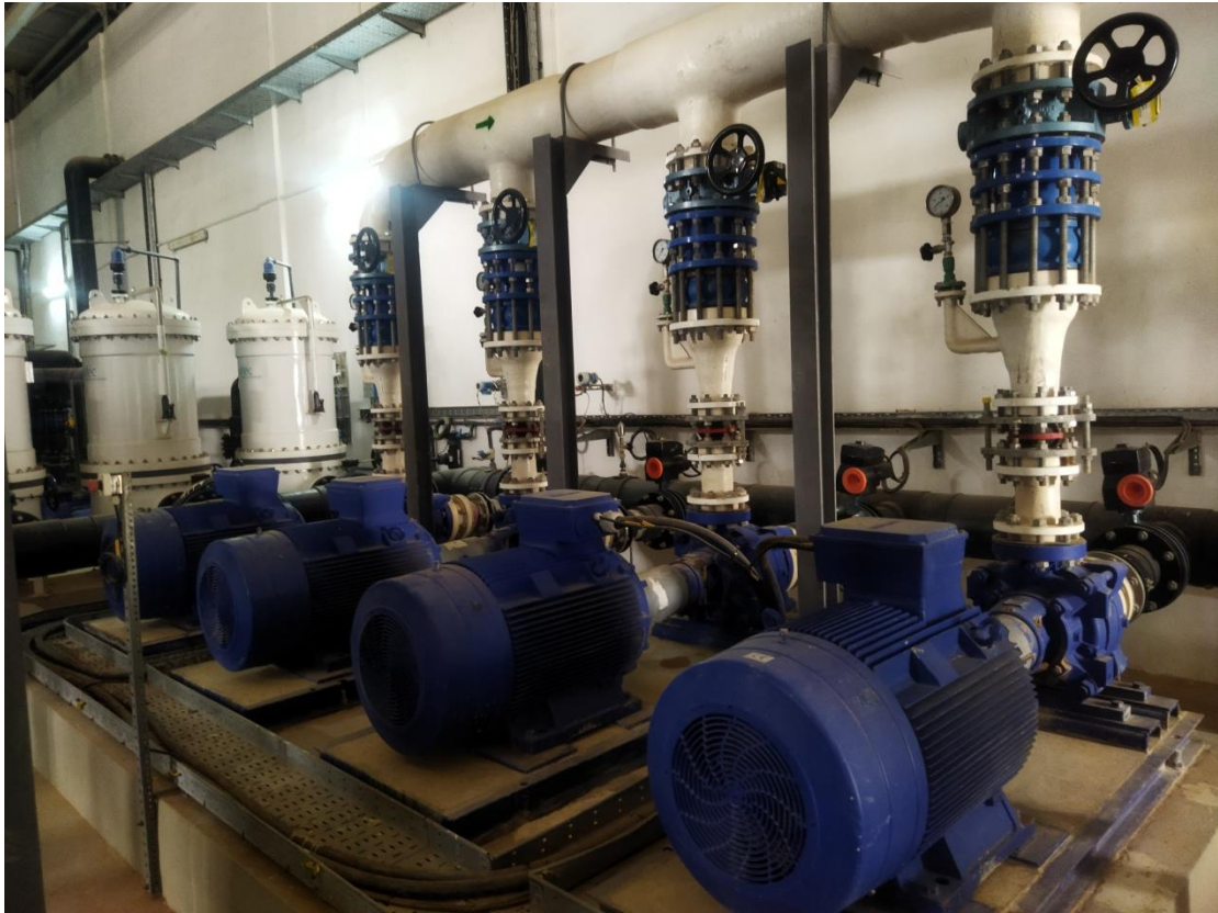
Figure II-8 : High pressure feed pumps
