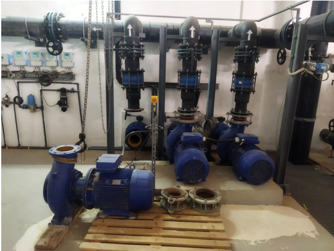
Figure II-5 : Low-Pressure Feed Pumps
