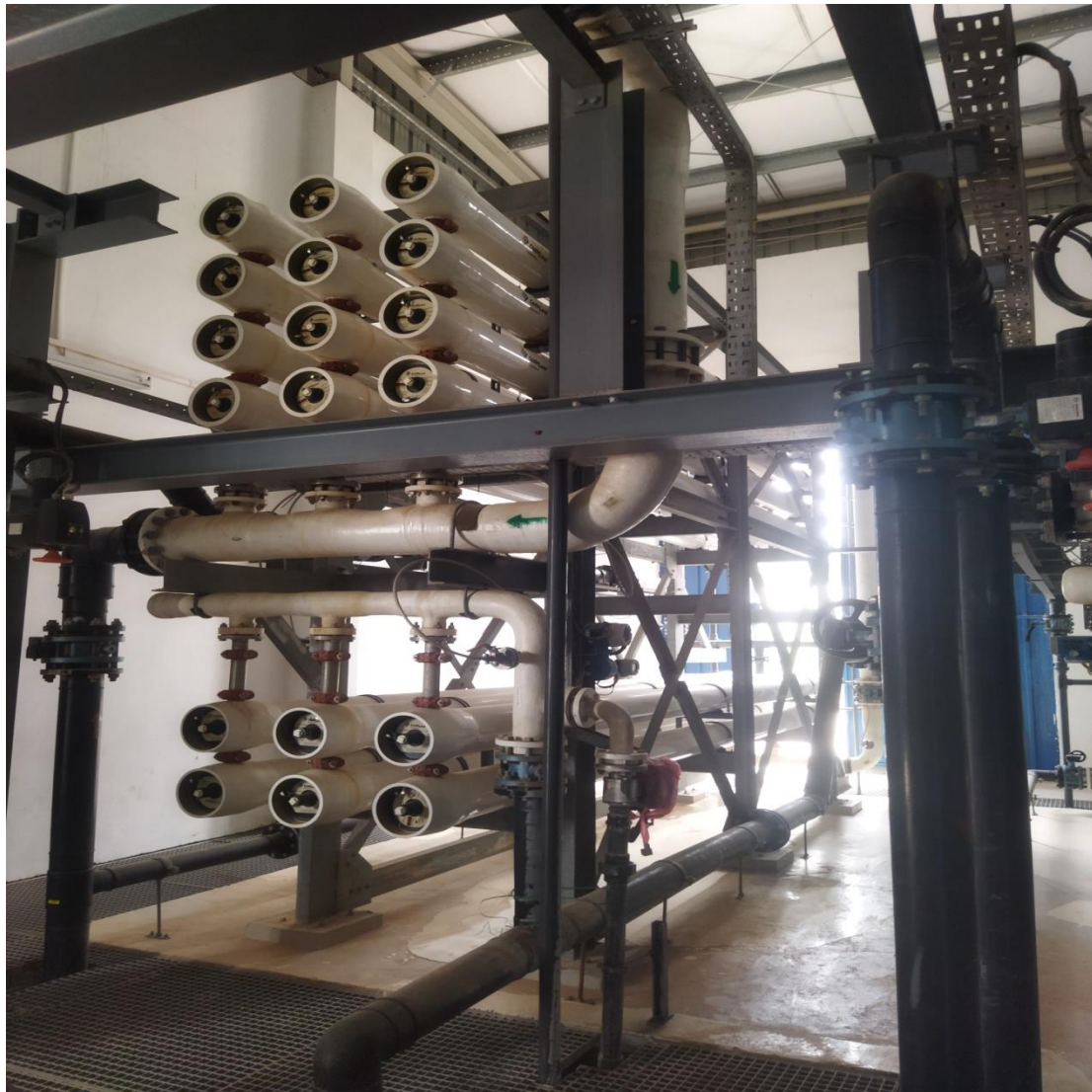
Figure II-12 : reverse osmosis line
