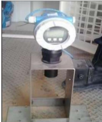
Figure II-13: Tank level sensors
