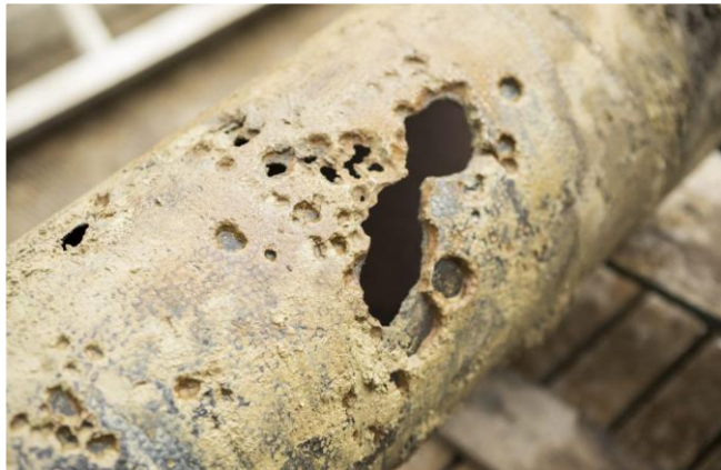
Figure I.2 : Corrosion caused by mercury in gas pipeline
