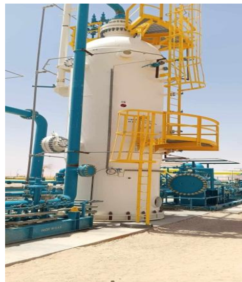
Figure IV.4: Mercury removal vessel
