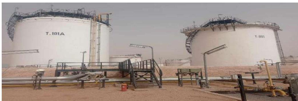
Figure 21 BAC DU STOCKAGE T-001 AND T-101A
