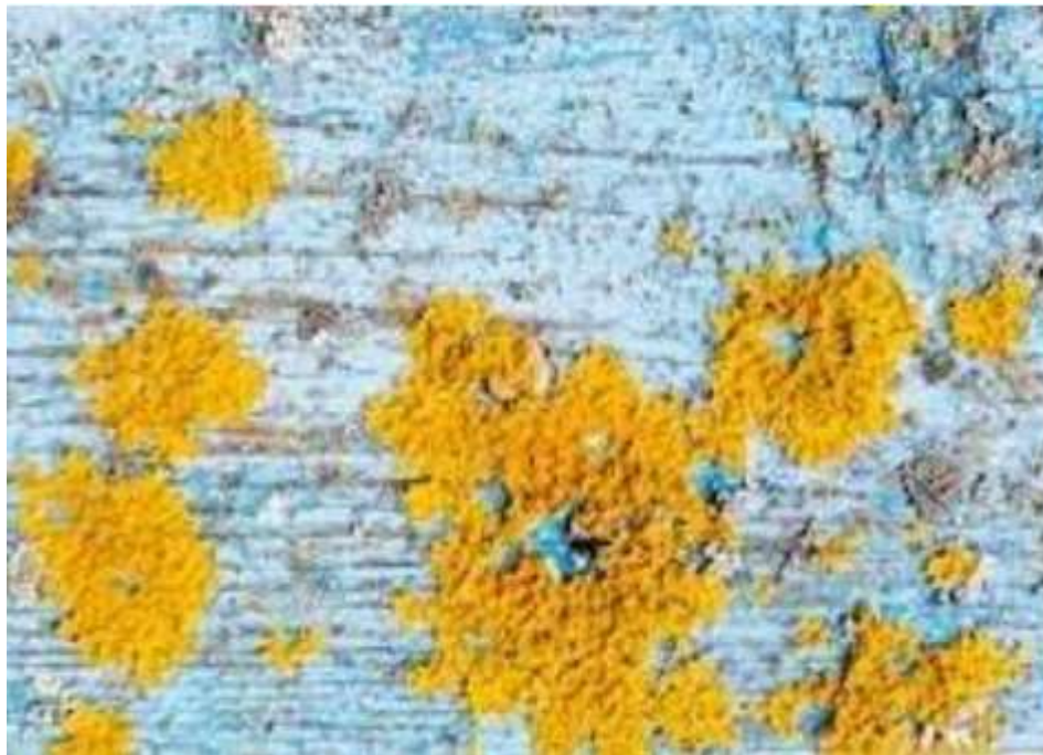
Figure I.2 photo de la biocorrosion.
