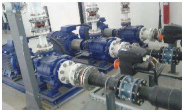
Figure III.9: pompe a haute pression
