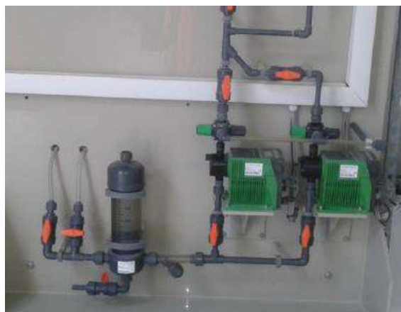
Figure III.7: pompe injection d'antitartre
