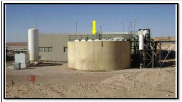
Figure 6: La cuve de floculation
