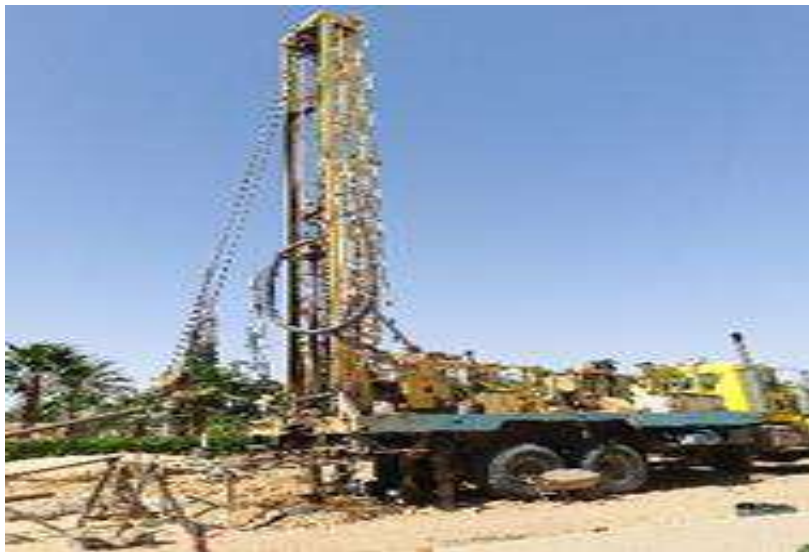
Figure II.04 : MAT de forage
