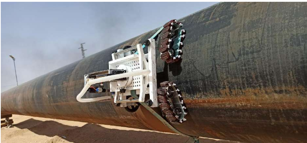
Figure 3.2: A photo of a welding robot being tested in the Algerian desert (Hassi Messaoud) 02.
