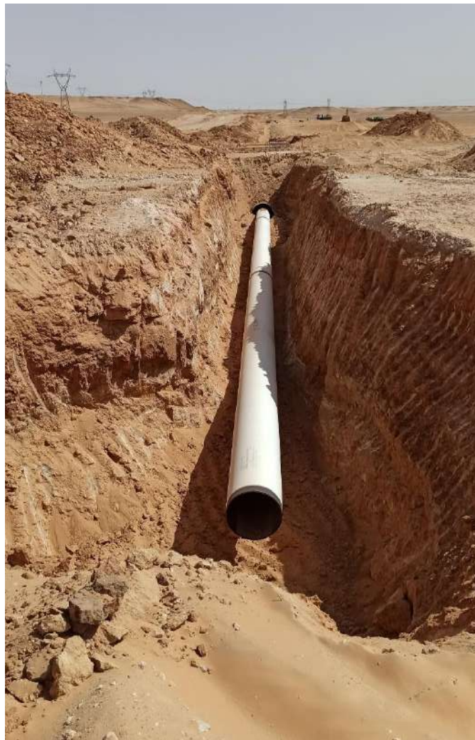
Figure 3.5: One of the risks and difficulties that exist in places where welding gas and oil pipelines.
