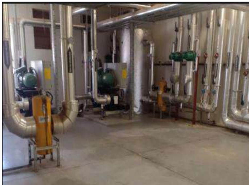
Figure II.15 ; Local PAC de maintenance installation fixe [19]
