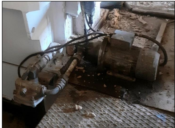
II. Figure 28: Oil Lubrication Pump.
