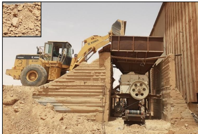
I. Figure 3: Primary Crusher.
