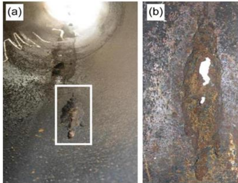
Figure II- 23: a) Corrosion b) Erosion
