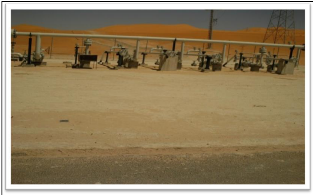
Figure I-10 : Gas Distribution Manifold
