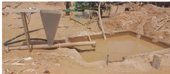
Figure II-8: Pompe de boue
