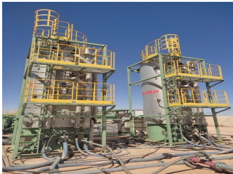
Figure III.16: colone de conditionnement
