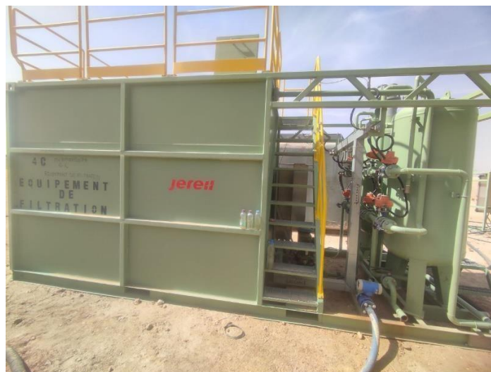
Figure III.23 : unite de filtration
