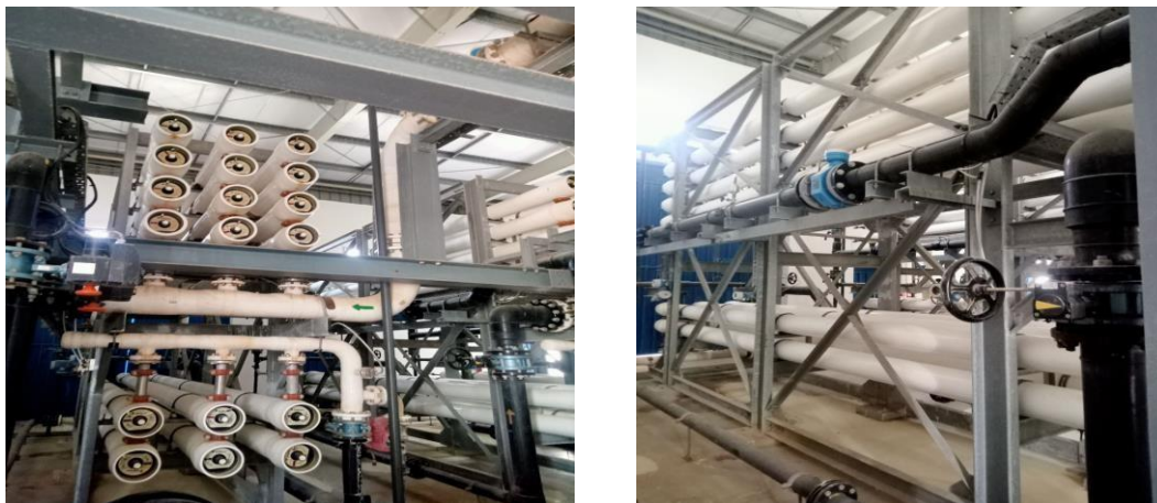
Figure III.05: Linge de membrane d'osmose inverse.
