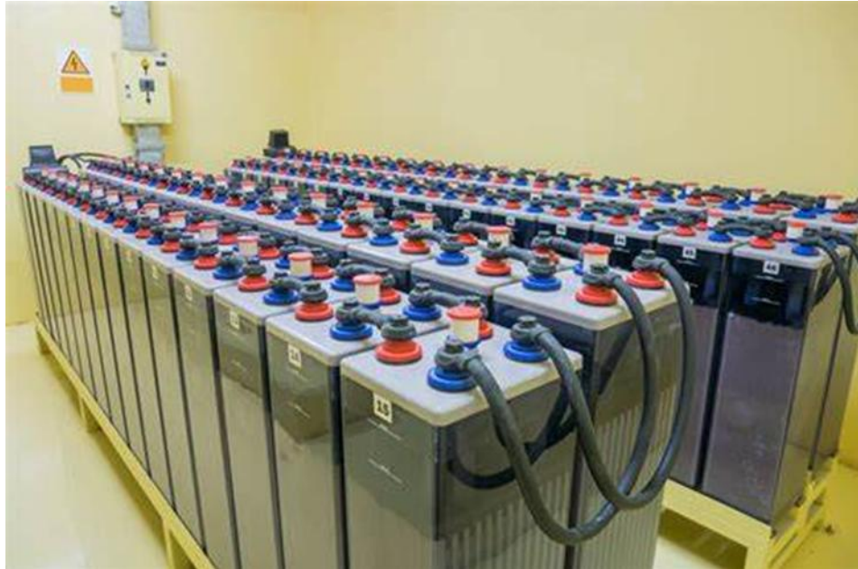
Figure 1.8 A group of batteries connected in series
