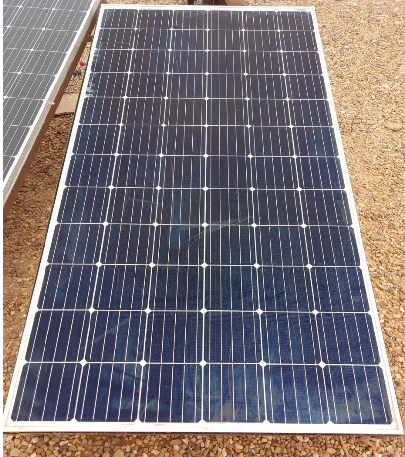
Fig III.10: Picture of the PV Panel.
