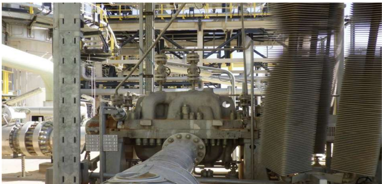
Figure II.5: pompe centrifuge 103-PA-023B
