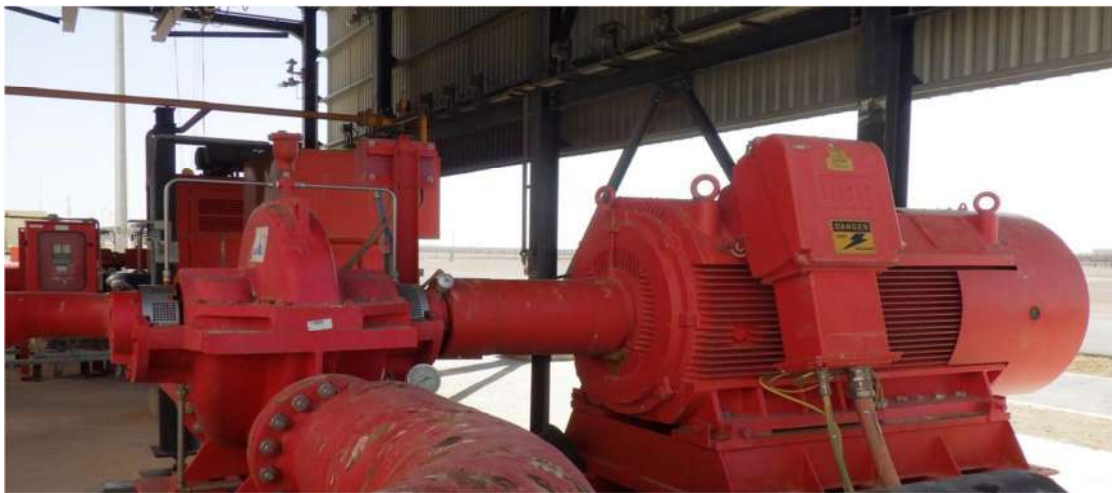
Figure II.4: pompe anti incendie 402-PA-002A
