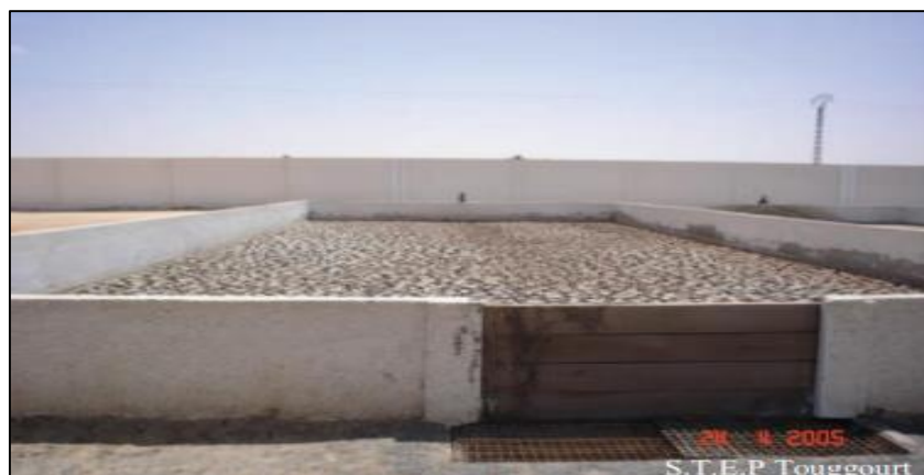
Figure 08. Sludge drying bed in the Touggourt station (Ghettas,2008)
