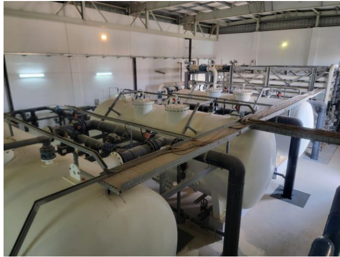
Figure 0-3 : Sand filtration tanks
