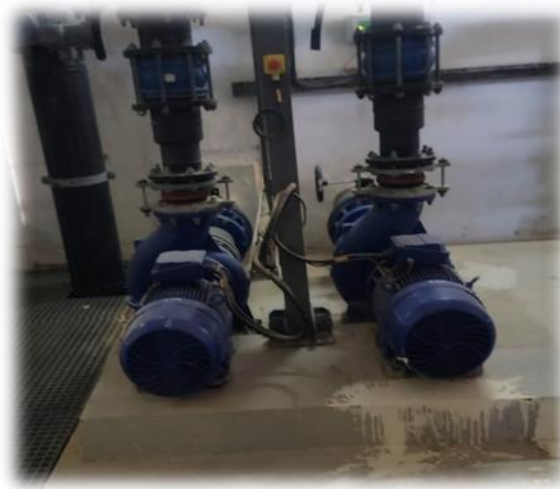
Figure 0-15 High Pressure Pump (HP)
