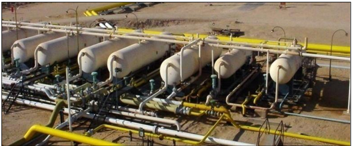
Figure I.7 : Bac de stockage [1]
