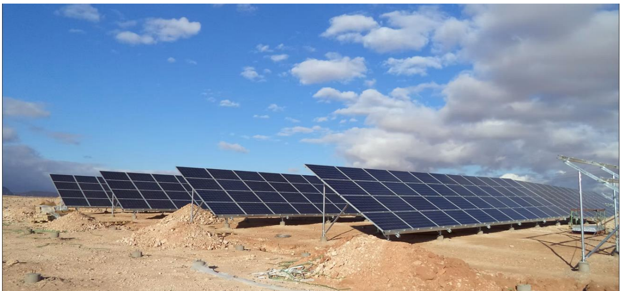
Fig I.2 Ain-El-Ibel - Djelfa - Solar Plants - 53MW – Algeria [13]
