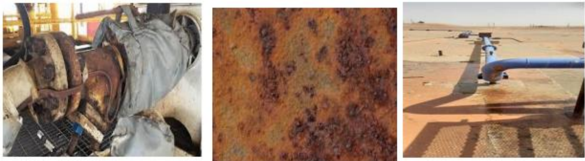
Figure III-1: Corrosion Of above-Ground Production Installations
