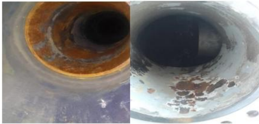
Figure III-2 : Bacterial corrosion of pipes
