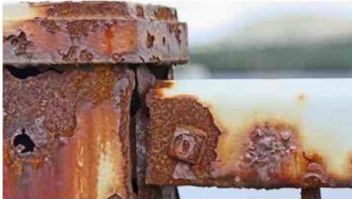
Figure I- 9: Stress Corrosion Cracking (SCC)
