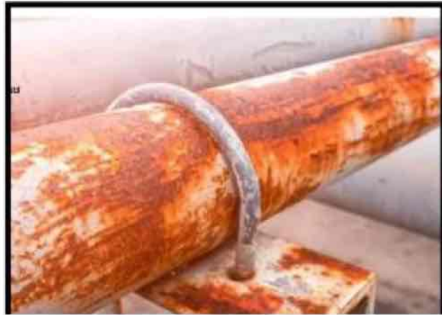
Figure I - 3: Uniform (General) Corrosion
