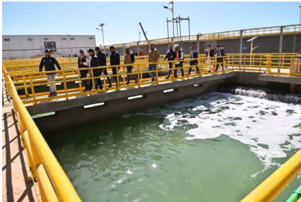
Figure 11:Hydraulic Systems: From Water Transfer Pipelines to Storage Reservoirs
