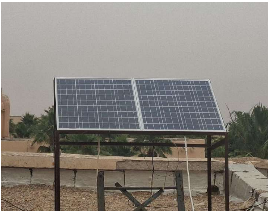
Fig 4.5: The 80 W PV panel.
