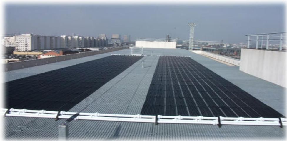
Figure I.7: Unglazed liquid flat-plate collector [14]
